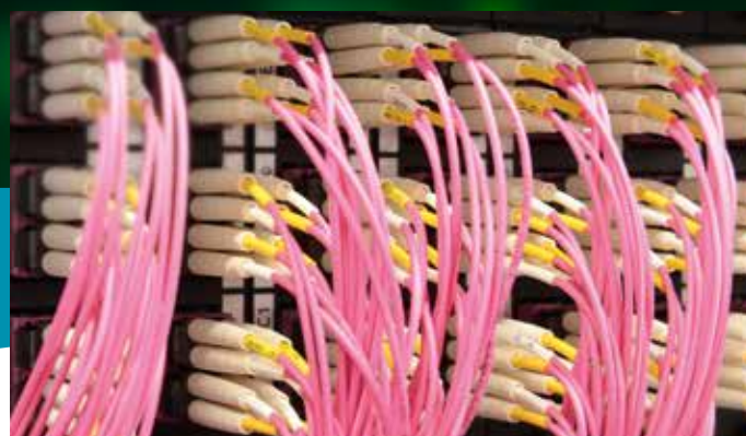
DATA CENTRE SOLUTION (DCS)
