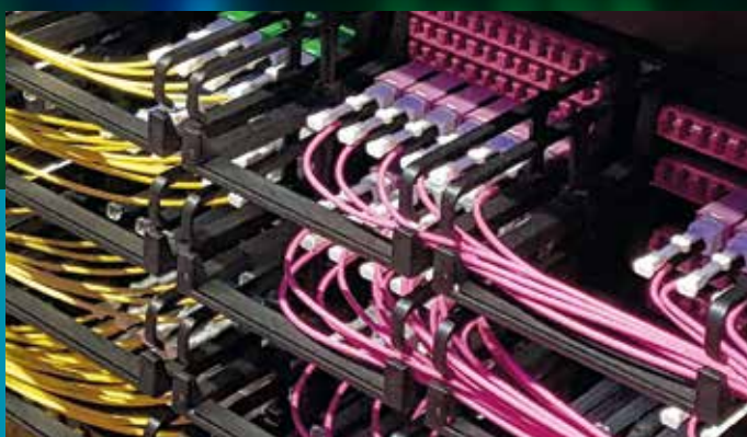
HIGH-DENSITY DATA CENTRE SOLUTION (HD-DCS)
