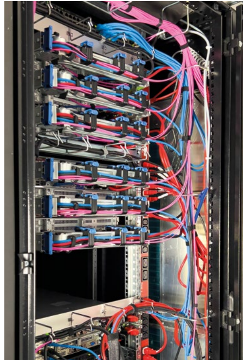
Redundant high-speed cabling in the rack
