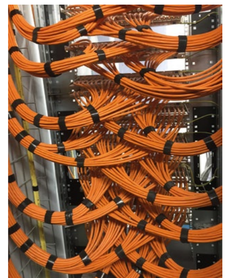
Network cabinet from the back side
