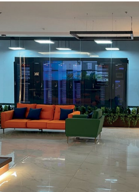
Energy efficient: the Smart Modular Data Centre in the MWAN head office
