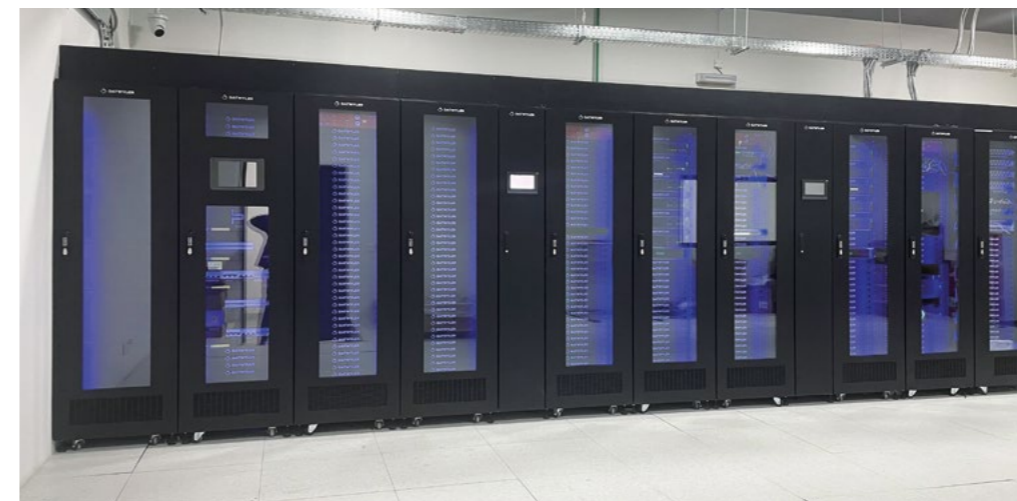
The new data centre at the company's head office
