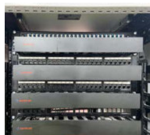
Patch panel assembly in a rack
