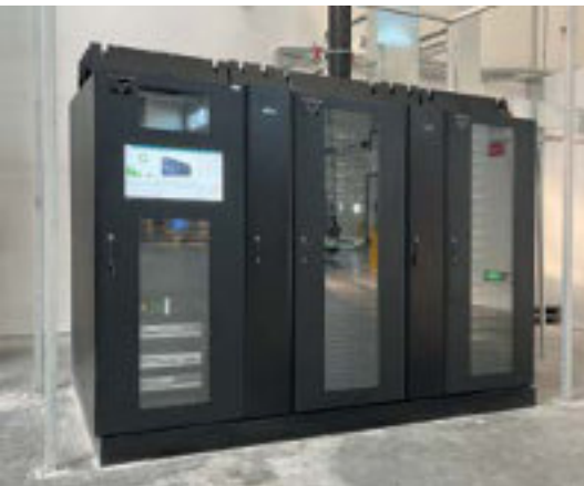
The data centre solution on the third floor of the new building
