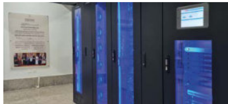
The Smart Modular Data Centre from Datwyler
