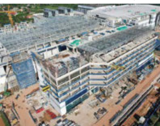
View of the construction site of the new AT&S factory in Kulim
